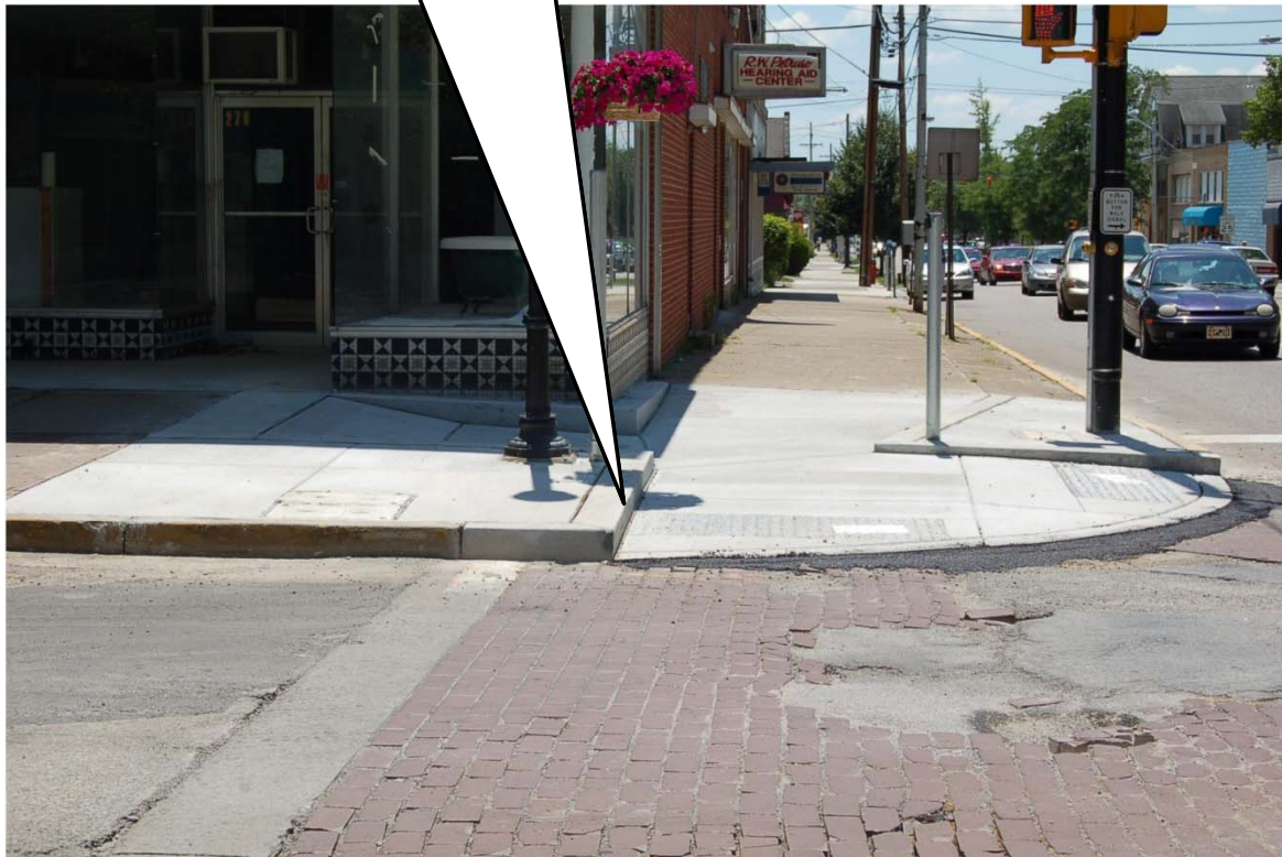
Poor Curb Ramp Design
